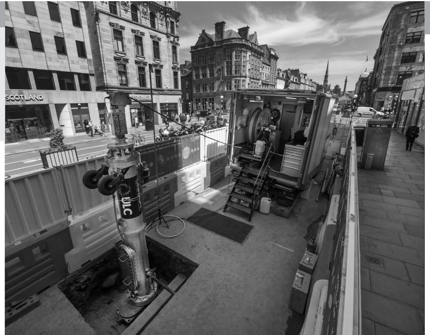
Not so new: In 2014 the London Borough of Camden piloted the use of robots to repair more than 50 gas mains joints for the National Grid
